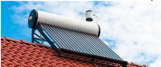
Figure 3: Renewable Energy solutions solar heaters
